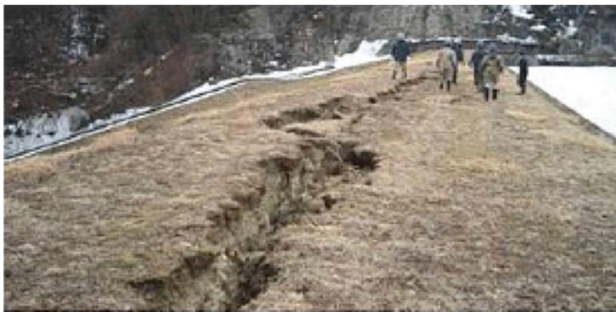
Fig. 47 Crack at the crest of the earth-filled dam (Kobayashi 2018)
