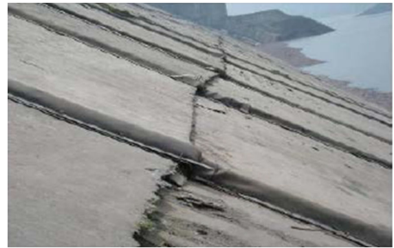
Fig. 20 Concrete slab dislocation Zepingpu dam during the Wenchuan earthquake (Kong et al. 2010)
