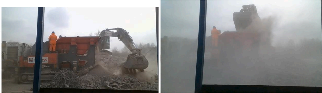
Fig. 4. Observed dustiness around the crusher.
